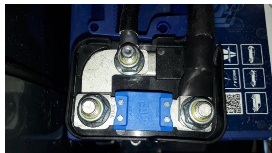
Box "A": starter motor fuse (Starter)
